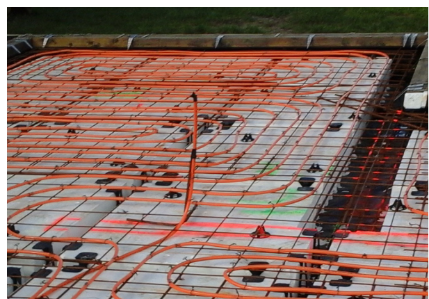
— Floor probe conduit run under the mesh from a wall to its final location in the floor in a Kiwi slab type underfloor heating system
