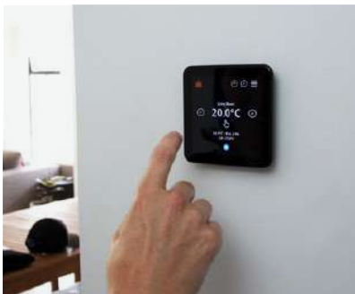
Running the System
